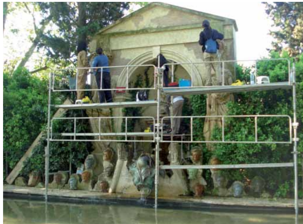
1 Restoration of the Caryatids of the Púbol swimming pool fountain Restauration des Cariatides de la fontaine de la piscine de Púbol
